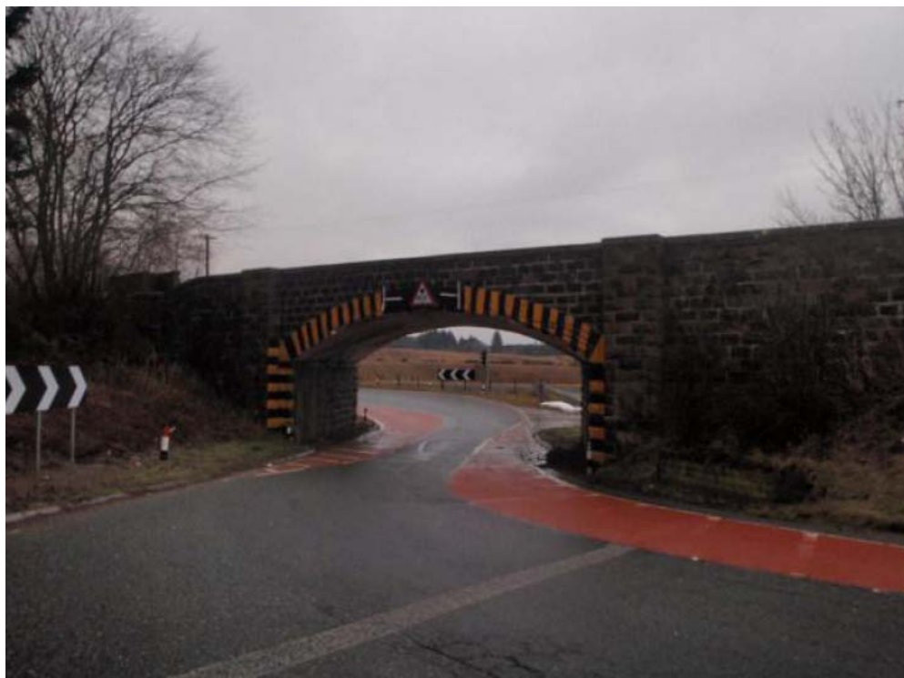
Photo: view through UB 293/084 in direction from Aberdeen to Inverness (DN direction)
