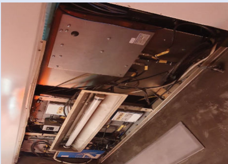
Equipment installation area in carriage roof
