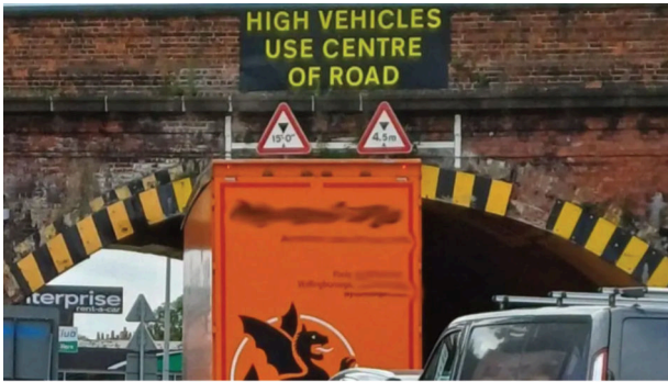
Harlaxton Road bridge, Grantham - struck 18 times in 2024/25. Perhaps not the most sensible signage! Photo: Network Rail
